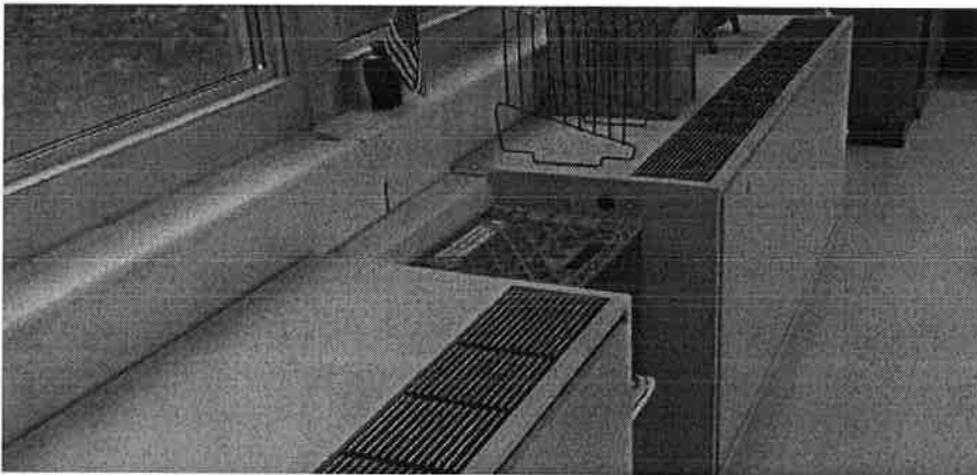
HVAC units in classroom
