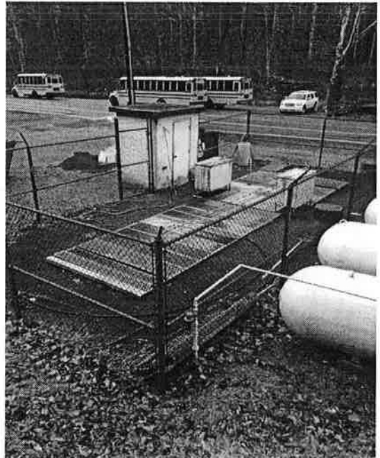
Wastewater treatment plant
