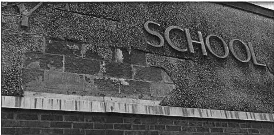
Exposed cmu at damaged façade panels
