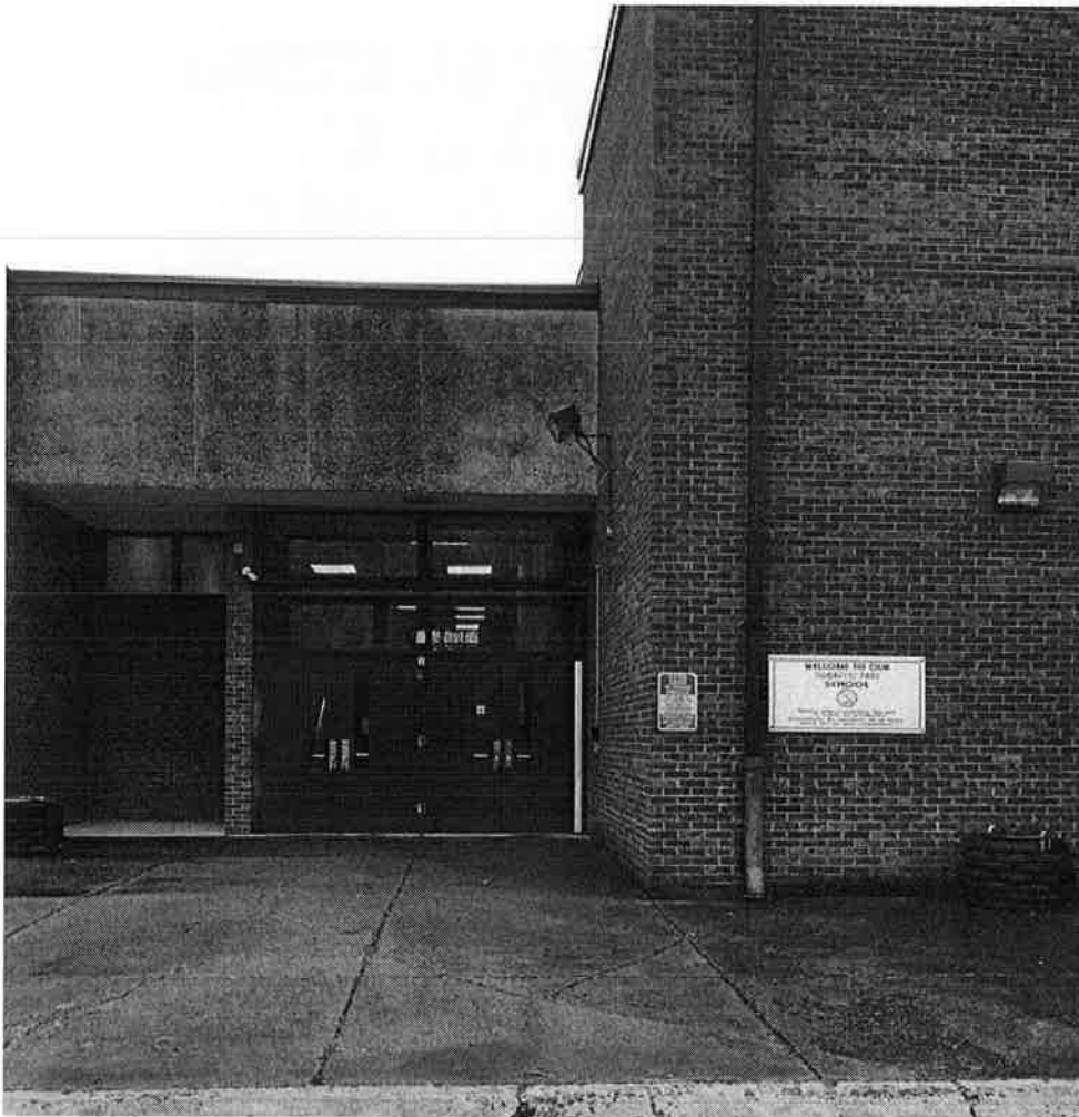
Worn façade panels at entrance
