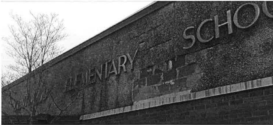
Damaged façade panels at front of school
