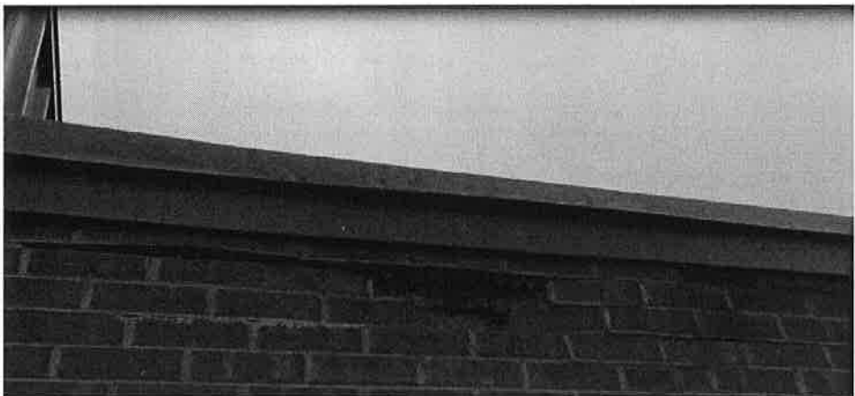
Damaged brick at roof
