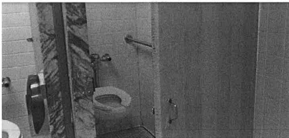
Restroom adapted for handicap use does not meet current standards
